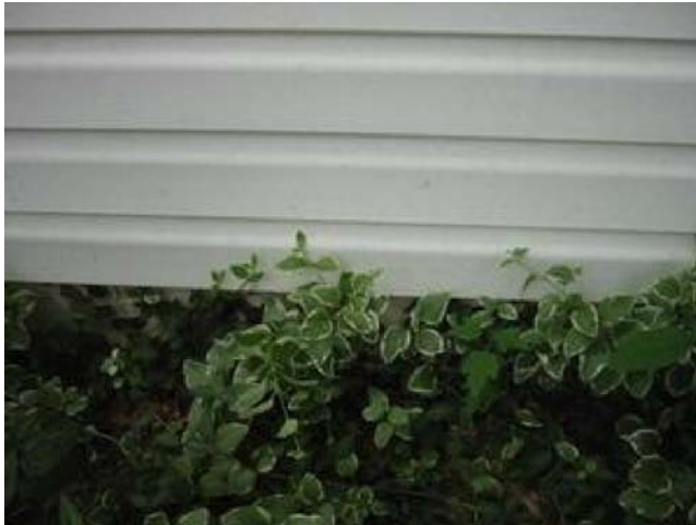
Ivy growing behind siding.
